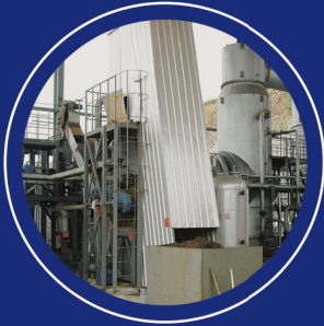
➤ Solid waste crusher
