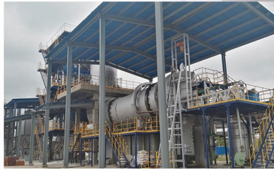
Fuse powder waste liquid and residue | 1.5t/h
